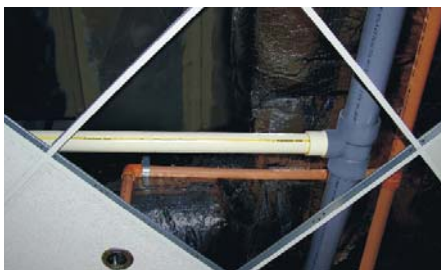
The Hilton Garden Inn® in Romulus, MI, was constructed using FlowGuard Gold® and Corzan CPVC® pipe and fittings for the plumbing system and BlazeMaster® CPVC pipe and fittings for the fire sprinkler system.
