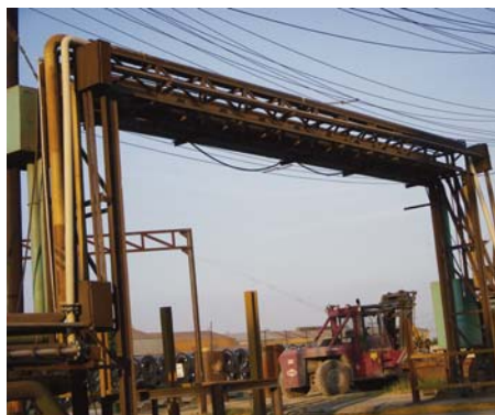
Large steel mill plant in Mexico replaces metal pipes with GF Piping Systems' PROGEF Polypropylene System because it is chemically resistant to aqueous solutions of acids, alkalis, caustics and salts, and to a large number of organic solvents.
