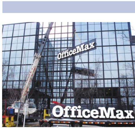
Installation, made easier with light weight properties of ACRYLITE® SignFlex sheet, required a combination of a bucket truck, ladder and crane trucks. Each letter contains 3/8" rivnuts, set within the letters' backs, that are installed with stainless-steel, threaded rod.
