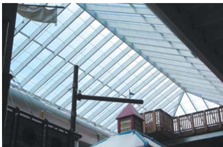
The material used in this skylight application was Gallina policarb 32 mm – 7 layers, clear.
