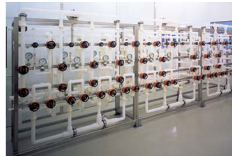
PVDF ultra high-purity water piping system
